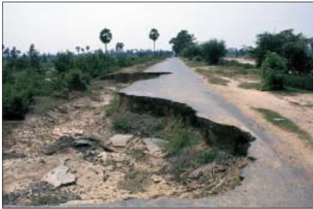
When flood-damaged roads and bridges are not restored quickly, transportation and shipping costs rise and with them, the prices paid by consumers
