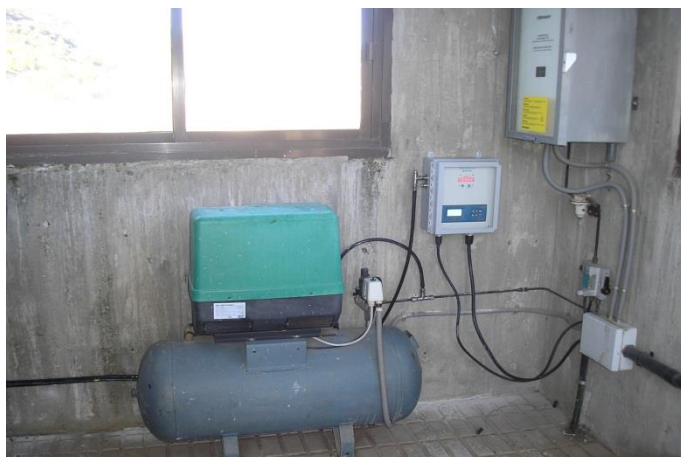
Reservoir level measurement system
